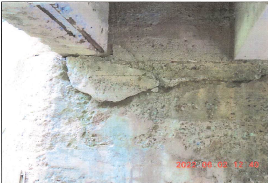
Photo 4: Cracking and Spalling on East Abutment Wall
