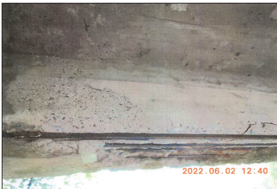
Photo 8: Spalling on North Exterior T-Beam
