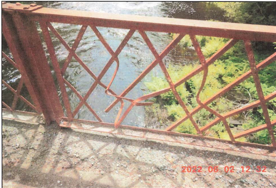
Photo 9: Deformation on South Barrier
