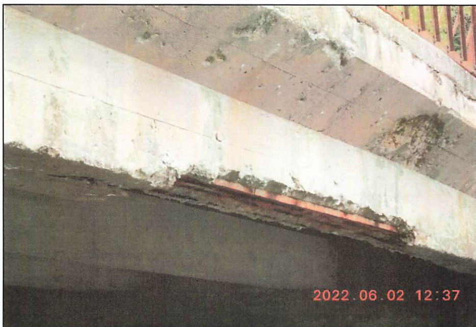
Photo 7: Spalling on South Exterior T-Beam
